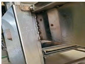
Lumpy welding joints can be areas of harborage. Photo credit, Audra Bissett
